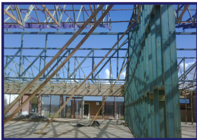
The Lakes College, North Lakes Structural & building hydraulic services for General Learning Area, Main Entry Pavilion, Roofed Walkway & Resource Centre.
